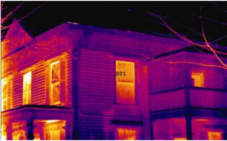
ABOVE: After insulation and air blocking, heat loss and air leaking is significantly reduced as seen in this infrared image.
